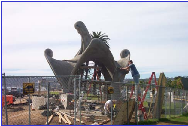
Kevin Dunwell and John Smith work on one of the four trellis columns
