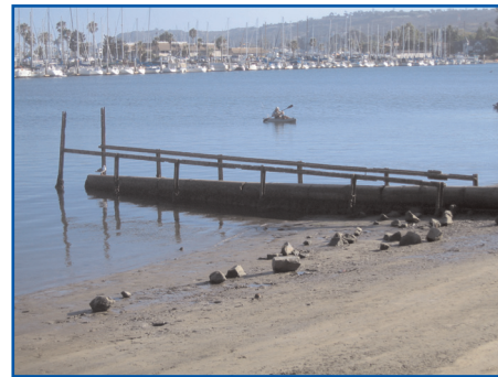
The outfall pipes are located at the foot of Bessemer and north of Qualtrough. Above is the pipe at Bessemer.
