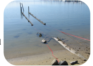
Both pictures show each storm drain as of September 16, 2009. Work had begun!
