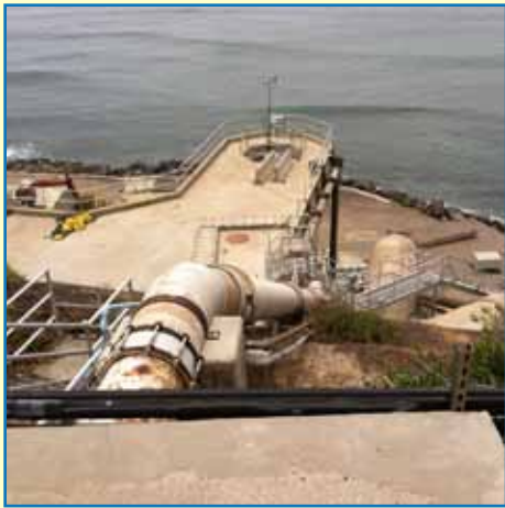
The beginning of the 90-foot drop to the ocean. The outfall produces hydroelectric power.
