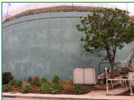
One of the seven on-site digesters
